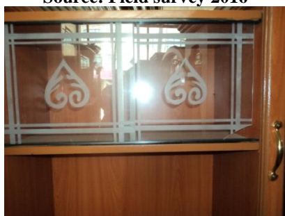
Figure 12: Broken glass. No intention of repair Source: Field survey 2016
